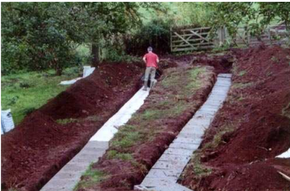
Figure 2. The trenches are now both covered by the slabs and the geotextile is laid on the top.
