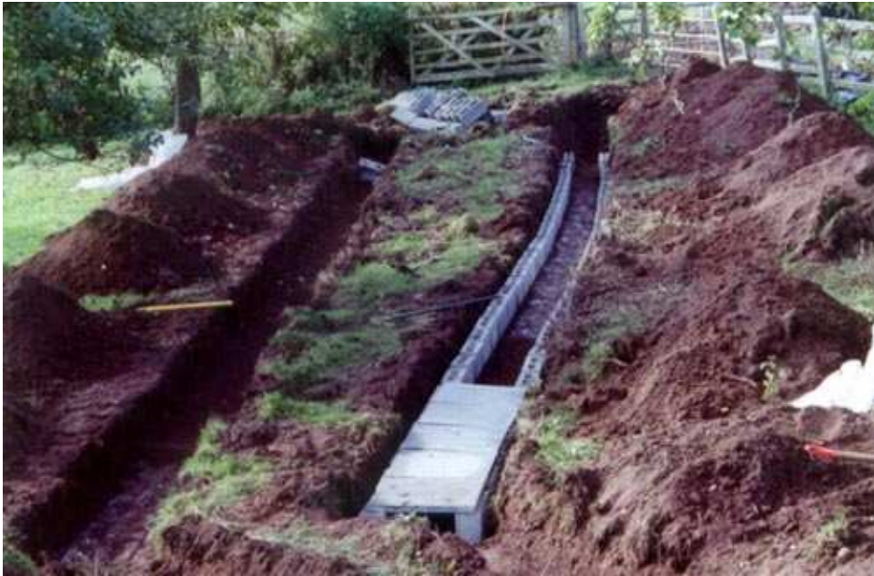
Figure 1 this system for a house has two parallel trenches. Both have been excavated and the bases have been laid so the first 6 metres fall at 1:20. The blocks have been laid with a gap of about 30 mm between them and the slabs lay on the top. Please note that the base of the trench ahead of the slabs has been raked to avoid smearing and compaction.
